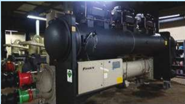
Picture 1 Change of water cooling machine to magnetic bearing cooling machine
